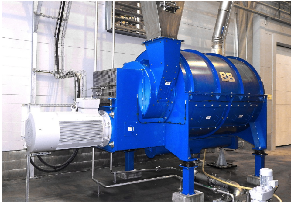
Figure 3.29. Photo Mechanical Dryer (Centrifuge)
